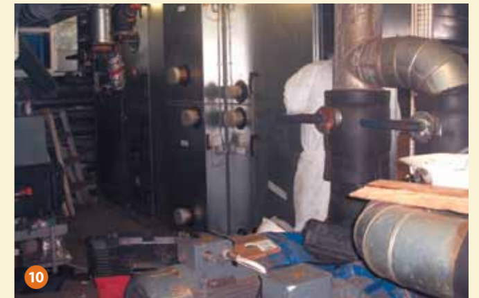
The new AHU is installed and the waterpipes will soon be finished.
