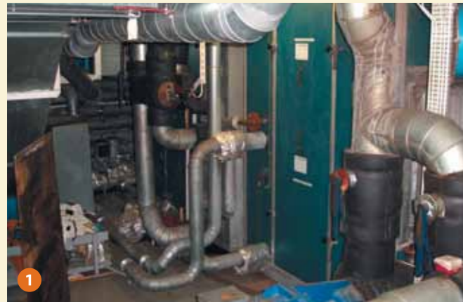
The room with the old AHU
